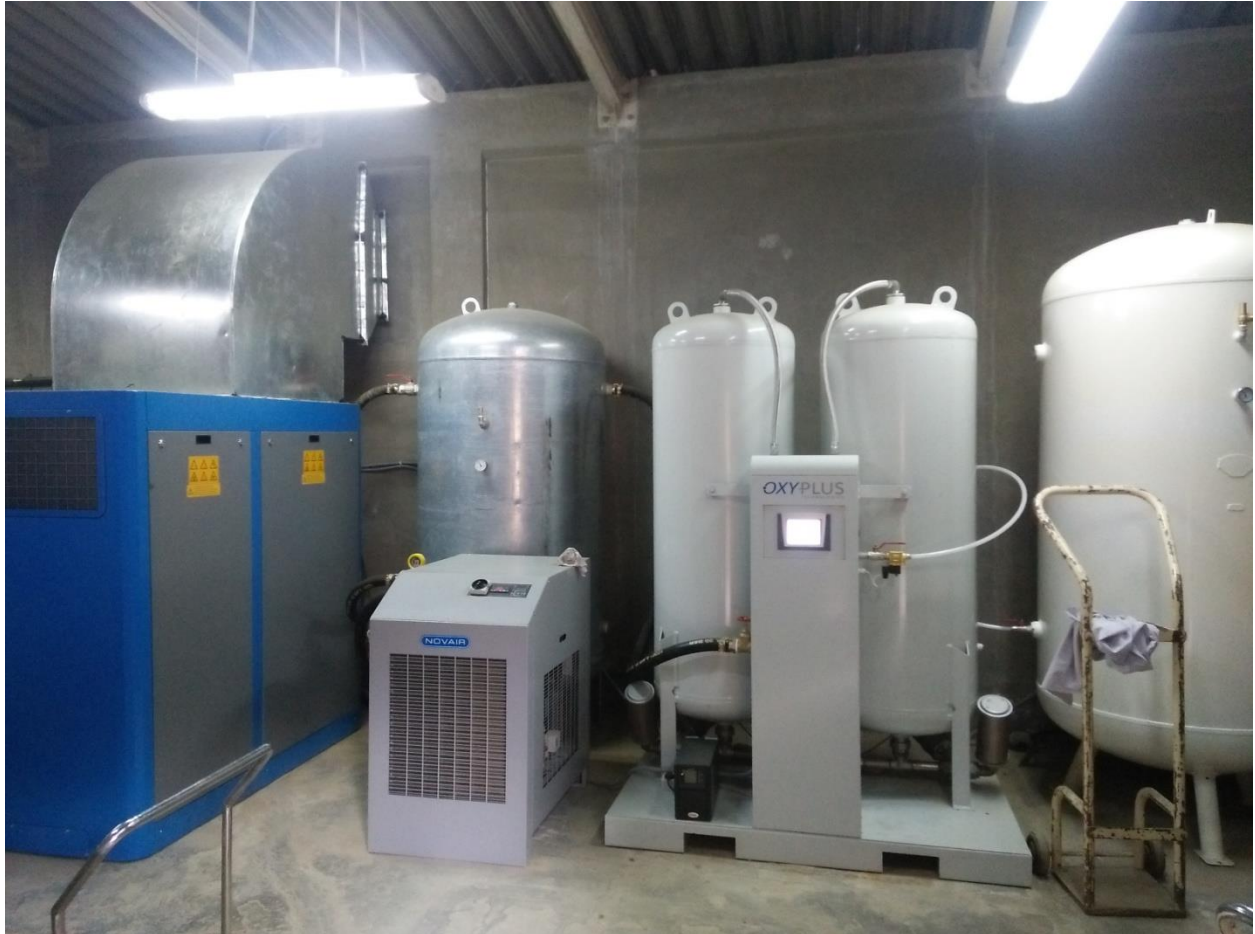
The new oxygen plant that was just installed by Medioxy PVT. LTD
