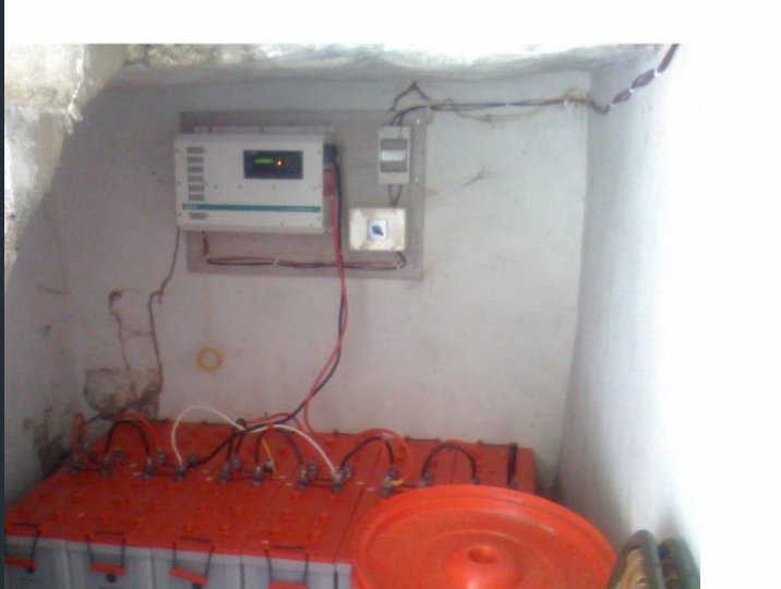
Inverter and battery system from Lotus Energy
